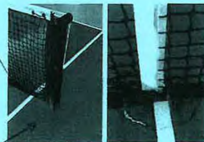
Cracking at Concrete/Asphalt Joint
