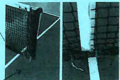
Cracking at Concrete/Asphalt Joint
